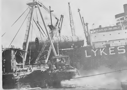
THIS STRIKING industrial photograph captures all the power and ingenuity that Mechanical Department riggers must utilize on the job daily. Lifting this 52-ton piece of equipment from the deck of a large freighter was considered one of the toughest rigging jobs handled in several years.
